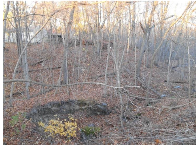
Figure 3: Additional view of eroded channel at Outfall 126, and bank destabilization.
